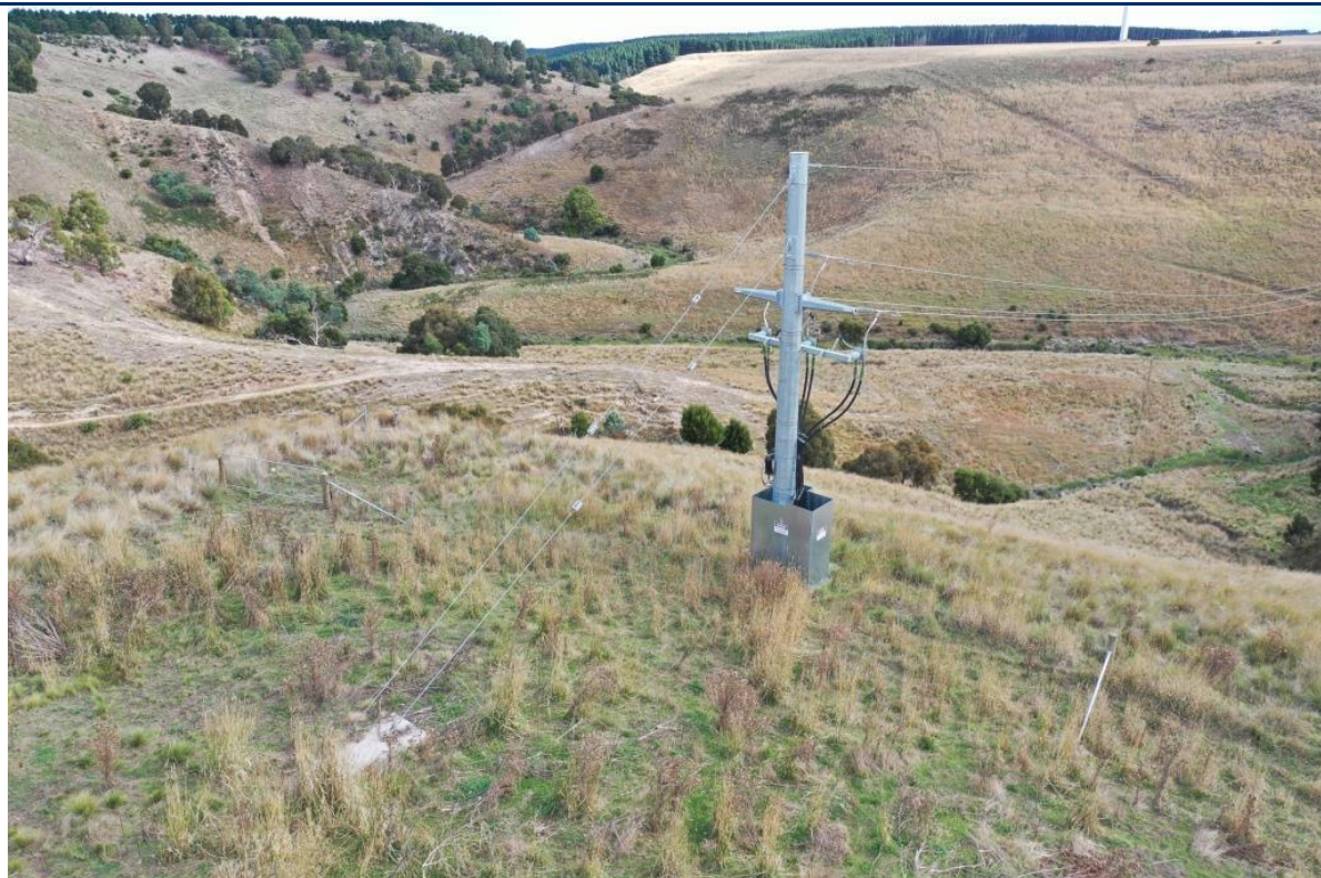
Plate 4 – Eastern Tower Structure - 33kV Overhead Line
