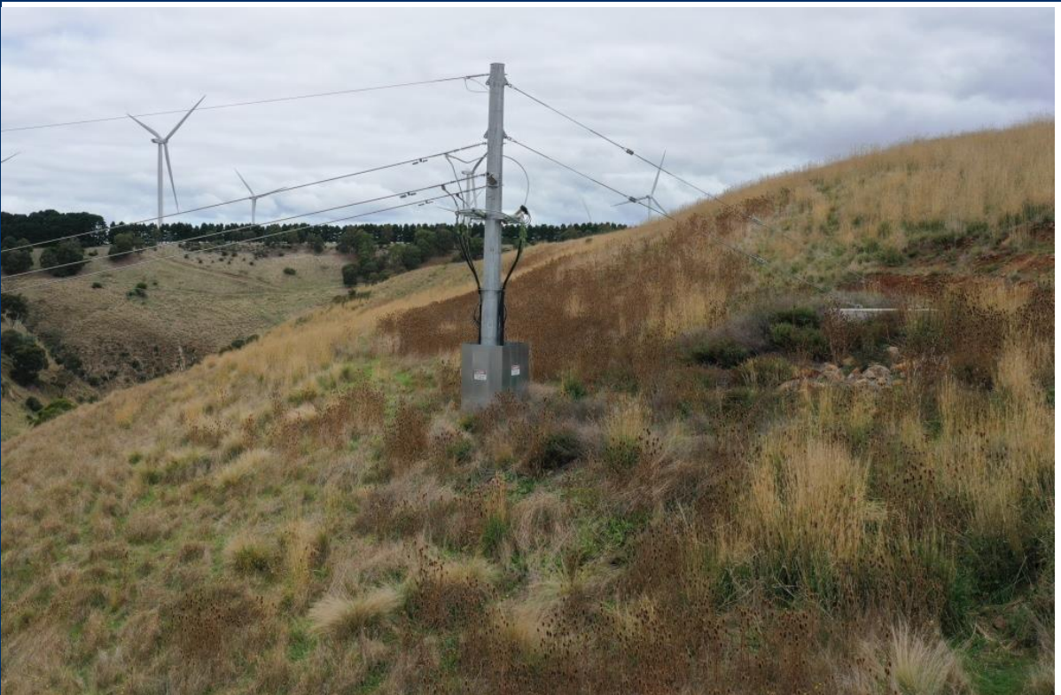
Plate 8 – Western Tower 33kV overhead line
