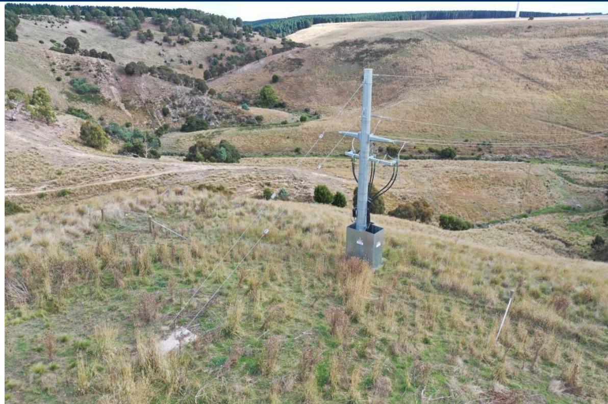
Plate 4 – Eastern Tower Structure - 33kV Overhead Line
