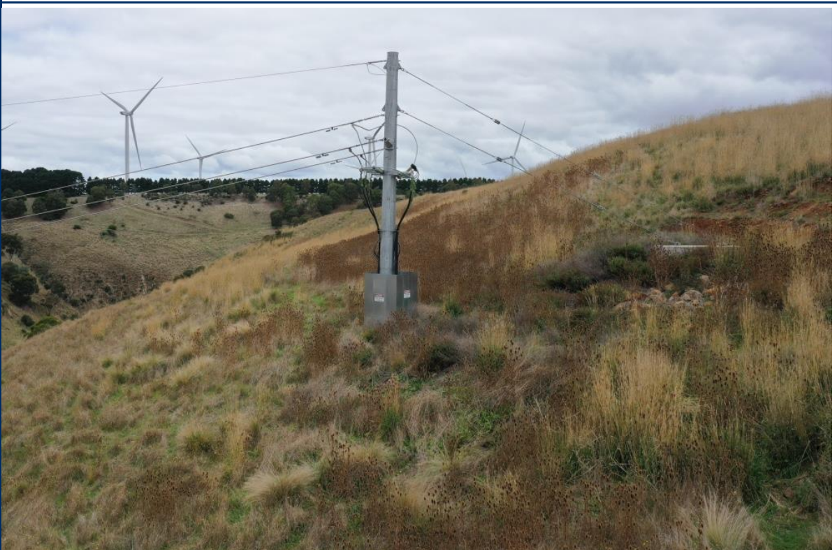
Plate 8 – Western Tower 33kV overhead line
