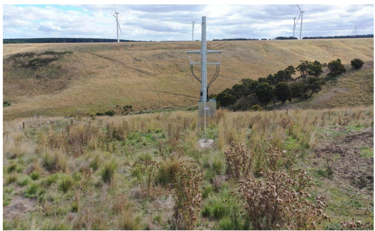
Plate 3 – Eastern Tower 33kV overhead line – View to west.
