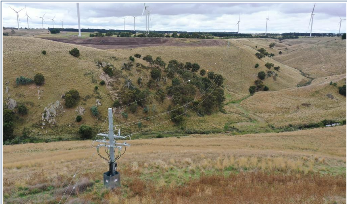
Plate 5 – Western Tower 33kV overhead line, View from south side of line. Aviation Marker Balls on conductors
