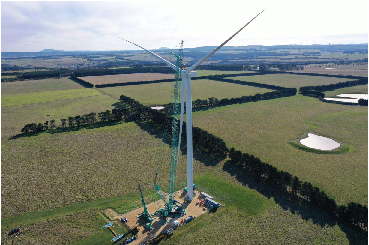
Erection of the first wind turbine in the South section of Goldwind's Moorabool Wind Farm.
