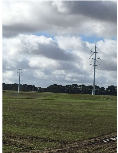
Figure 2 Image of the double circuit transmission line
